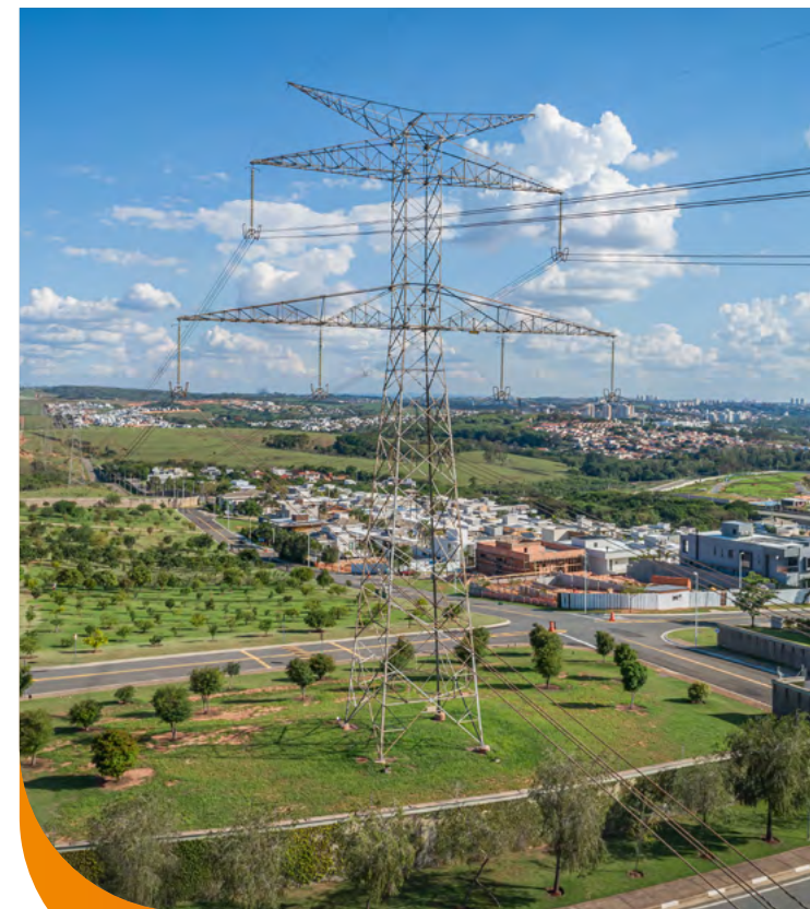
Transmission tower - Campinas - SP
