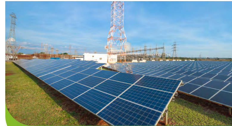
Tanquinho Photovoltaic Plant in Campinas - SP
