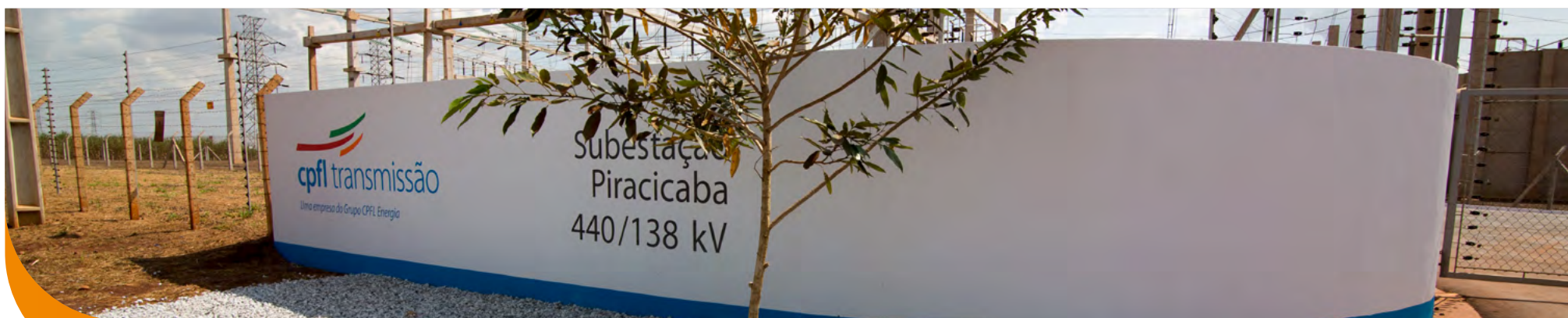
Piracicaba Substation - SP
