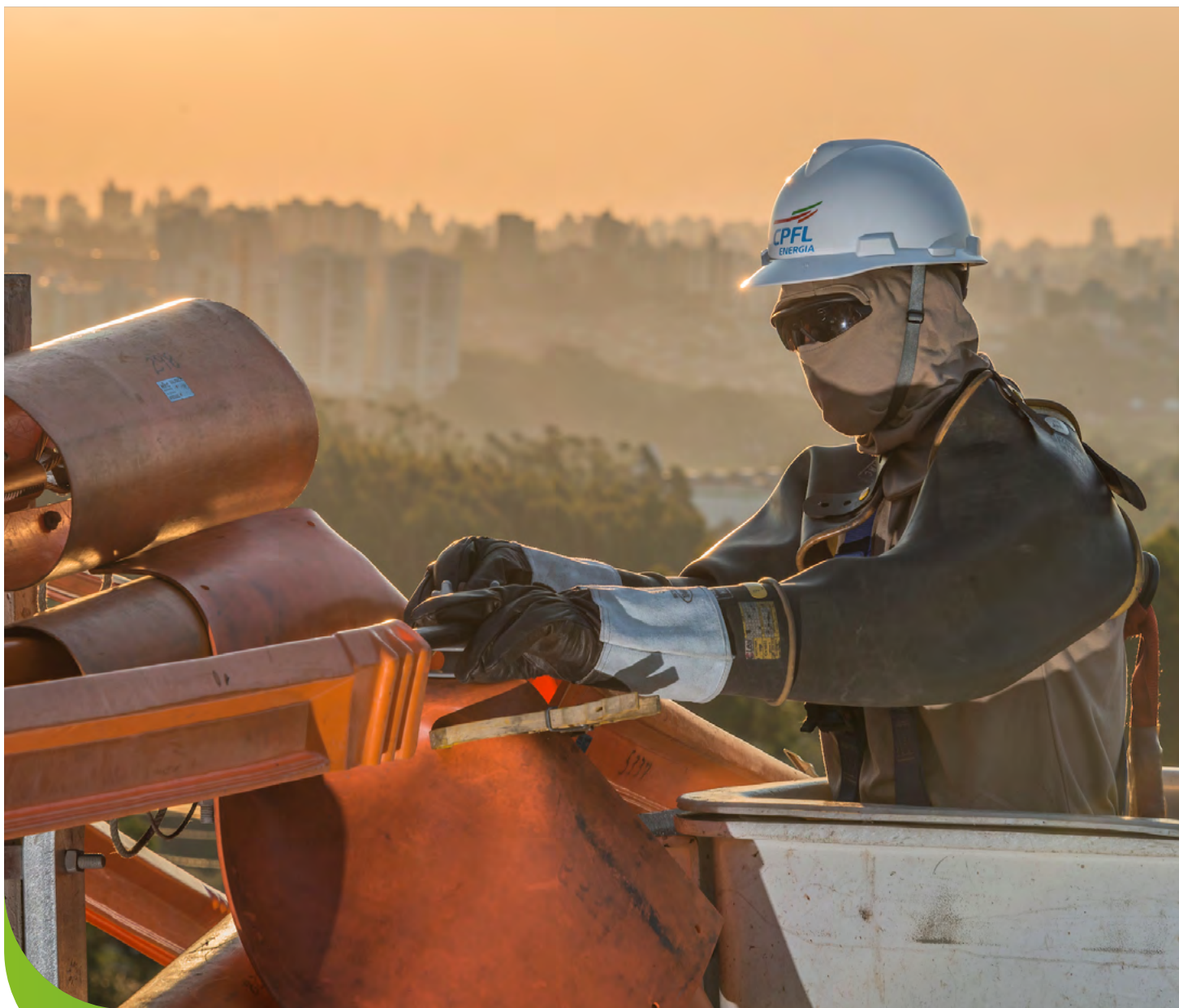
Employee at CPFL operation
