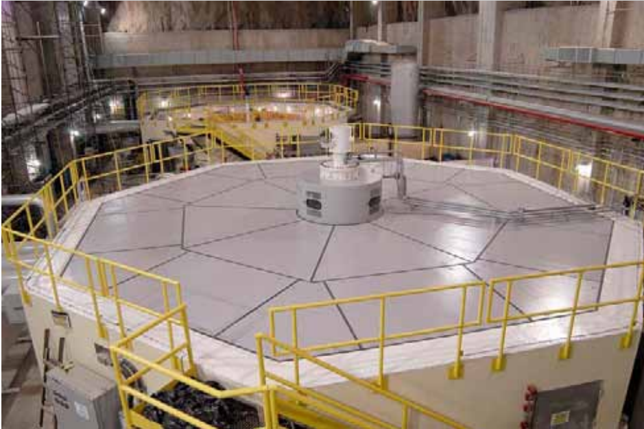
View of generator #01| Monte Claro hydroelectric power plant | Rio Grande do Sul
