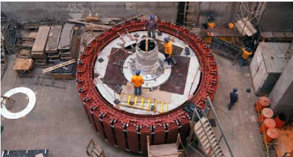
Installing the generator turbine | Barra Grande hydroelectric power plant | Santa Catarina and Rio Grande do Sul
